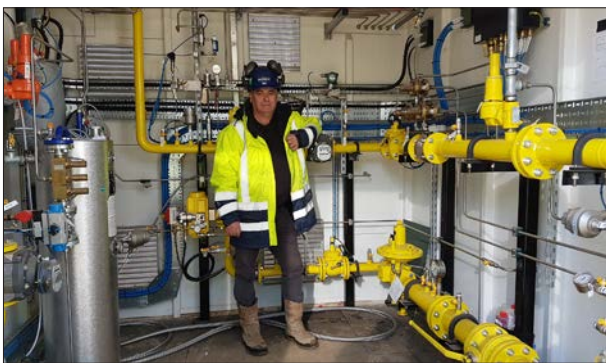
Plant manager Tim Wright is happy about the first gas delivery to the grid.
