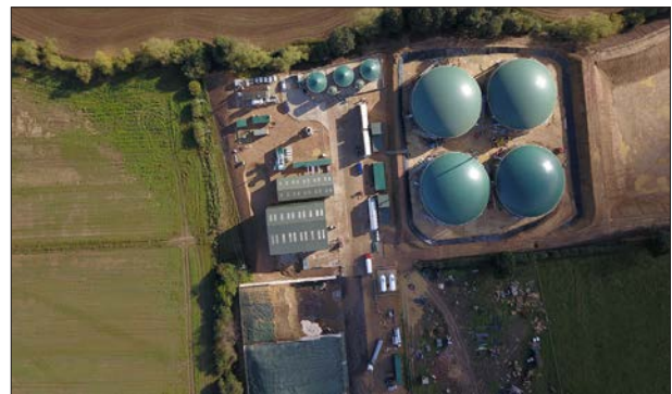
The biomethane plant delivers enough gas to supply about 9,600 households with green energy.
