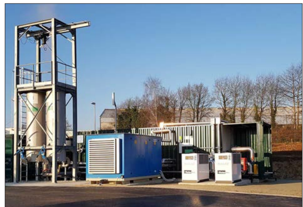
To condition the biogas into biomethane, WELTEC BIOPOWER integrated a membrane technology as a compact container solution.
