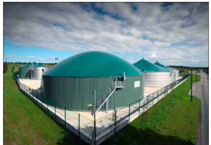
The two stainless-steel digesters in Aurora, each of which has a capacity of 3,573m 3 , will be fed with 100 tons of organic waste a day.
