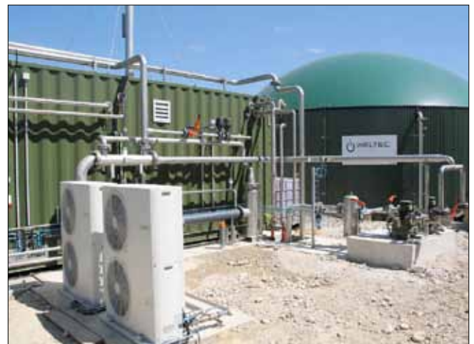
On 5 August, the „Longchamps“ biomethane plant in the Franche-Comté region in eastern France went live. Thus, 70 standard m 3 /h are now continually supplied to the natural gas grid of the French gas distributor GrDF (Gaz réseau Distribution France).
