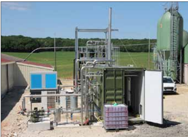
To ensure effective biogas processing, German plant manufacturer WELTEC BIOPOWER decided to deploy flexible, compact membrane technology.
